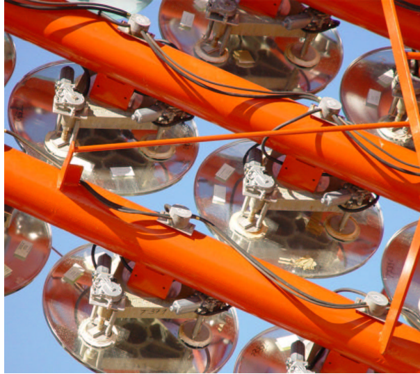
Fig. 17. Section of the dish showing mirrors, the mirror mounting brackets, the branch cable and the short connector cables.
